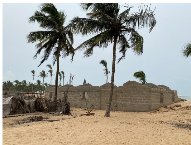
Figure 3. Destroyed classroom and sanitary facilities
